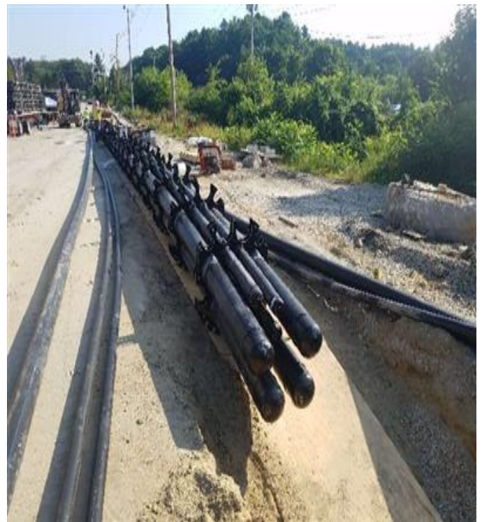
Fig 24: Assembling bundle before they install it in the HOBAS pipe. Viewing north. (7-29-19).
