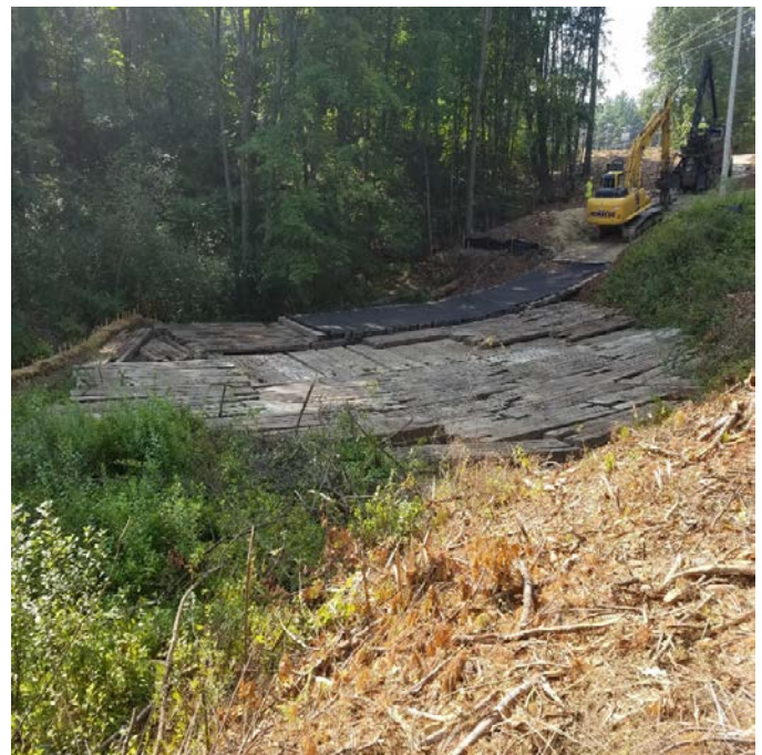
Fig 32: JCR installing timber matting and filter fabric around Str. 28, south of Oyster River. Viewing south. (7-31-19).
