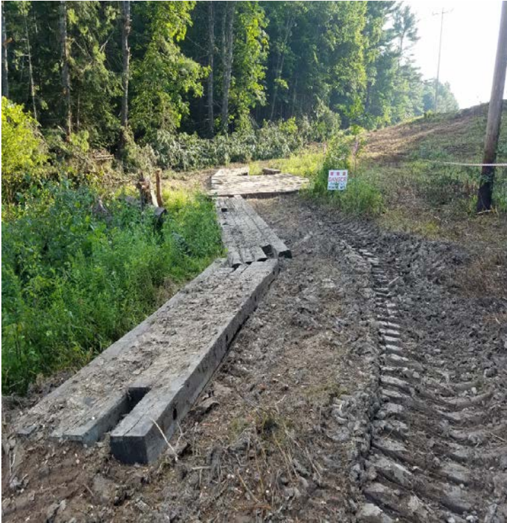
Fig 17: Access route between wetlands DW48 and DW50 (stream DS46 is down the slope to the left). Viewing north. (7-29-19).
