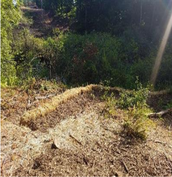
Fig 9: Combined straw bale and stump grinding berm, south of Oyster River. Viewing north. (7-26-19).
