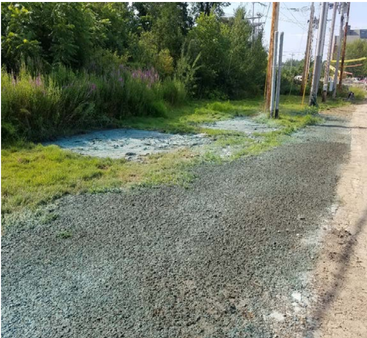
Fig 31: Restoration next to Colovos Rd where dewatering apparatus was installed. Viewing south. (7-31-19).
